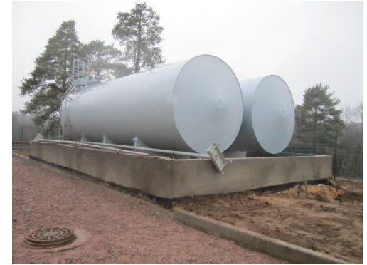
Water tank metallic
